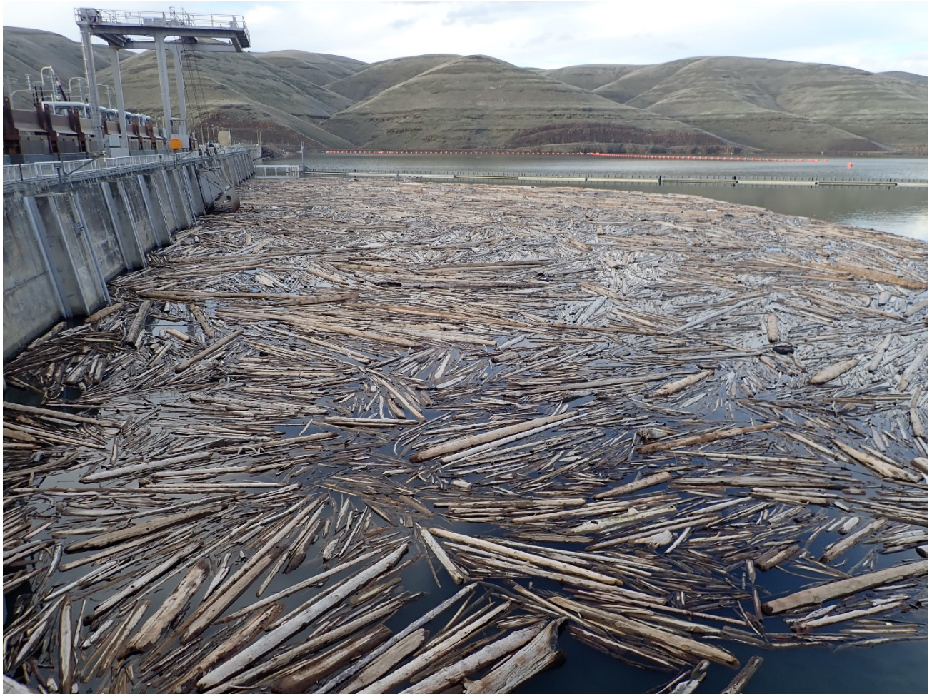
Image 2: Debris inside the trash-shear-boom at Little Goose; March 9, 2021.
